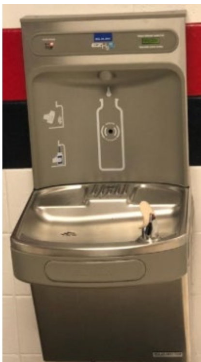
Water bottle filling station installed at Buffalo Prairie Middle School.
